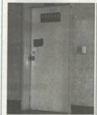
Poor condition of resting room
